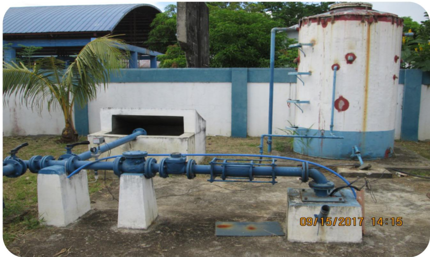
MARANA 3 rd PUMPING STATION
