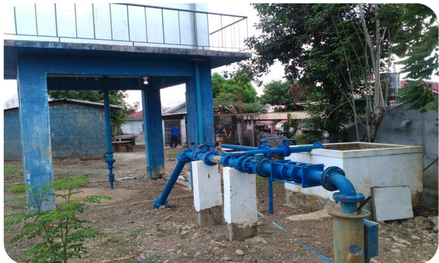
ALINGUIGAN 3RD PUMPING STATION
