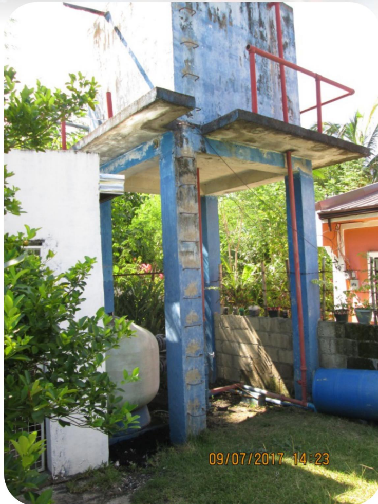
TREATED WATER STORAGE TANK
