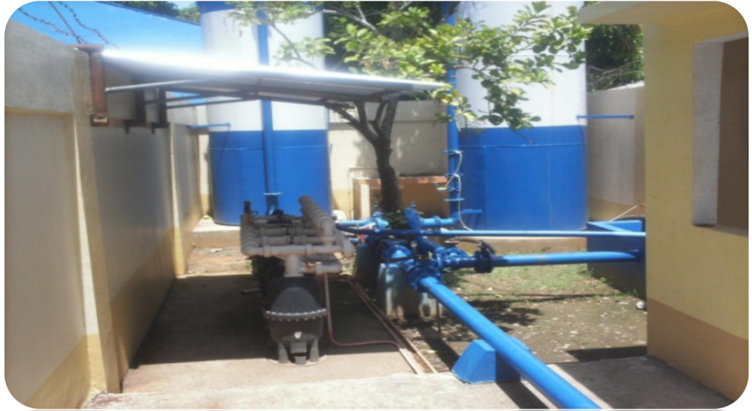
2 UNITS - COAGULATION TANK
