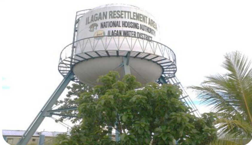
BLISS PUMPING STATION
