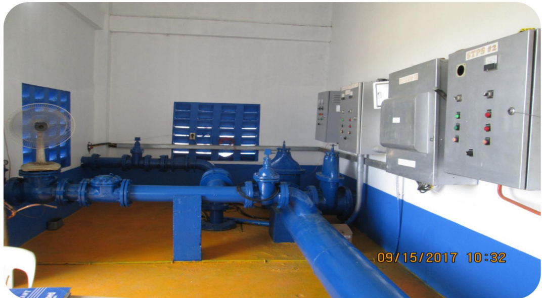
TREATMENT PLANT CONTROL ROOM
