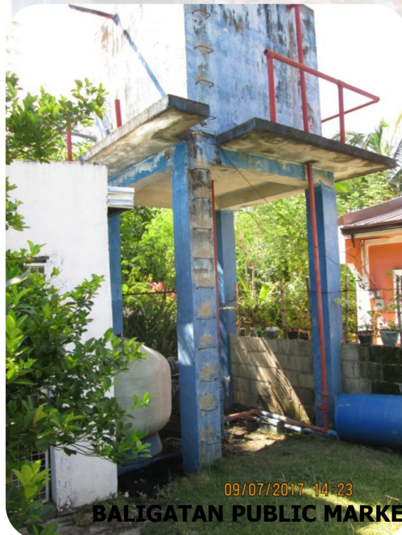
TREATED WATER STORAGE TANK
